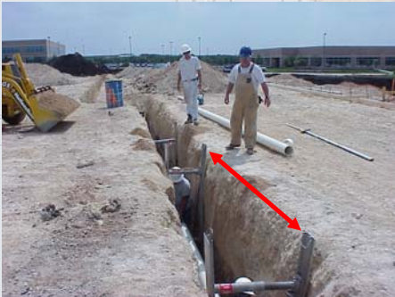
Developed under an OSHA Susan B. Harwood Grant, #46F4-HT01, by the Associated Builders and Contractors-Central Texas Chapter
